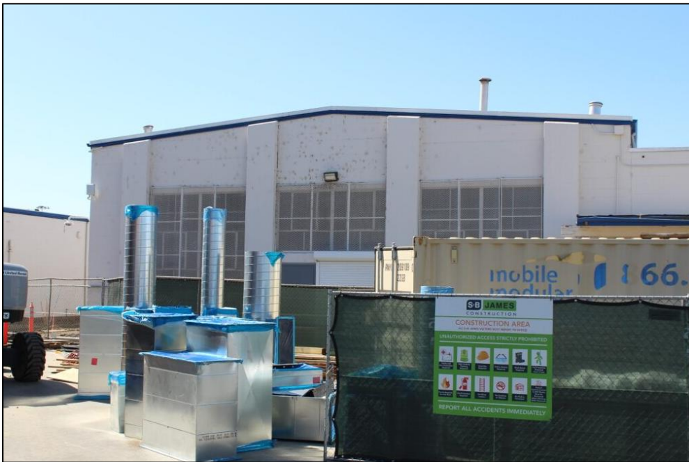
Photograph 18. View of the north (front) façade of the Shop #1, facing south (H. Fuess, 2025).
