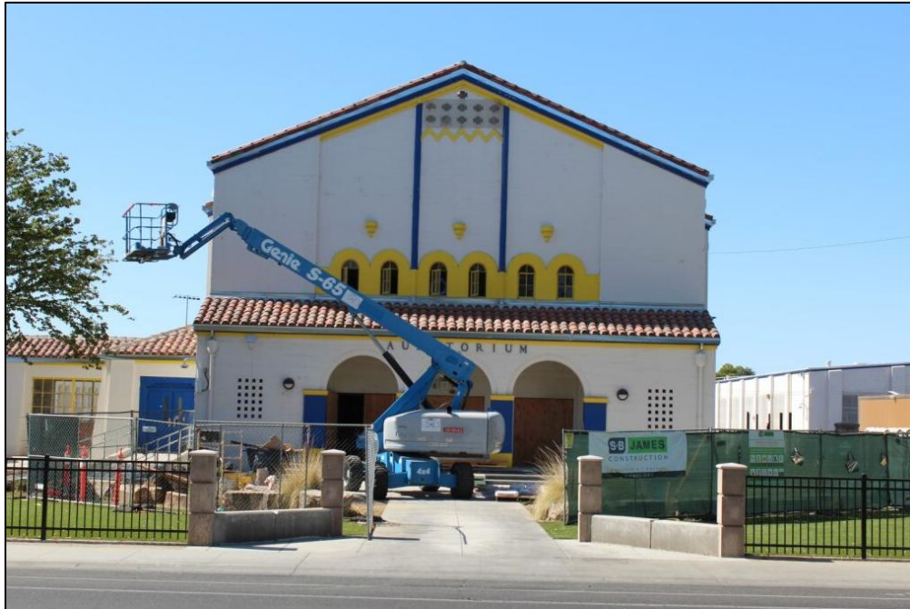
Photograph 13. View of the north (front) façade of the Auditorium, facing south (H. Fuess, 2025).
